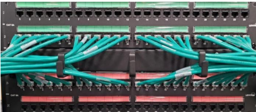
Practical use of 49253-LPM. 24 Patch Cords (6.0mm O.D.) per end. Cords route into Cable Manager from lower row of top Patch Panel and upper row of bottom Patch Panel 24 cords = 27.1% Fill Ratio for the 49253-LPM ring.
