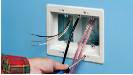
2 Pull cable. Insert box in hole. Tighten mounting wing screws to hold box securely against wall.
