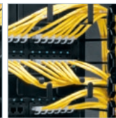
internal vertical cable manager
