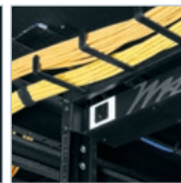
bracket for top cable pass-through between enclosures
