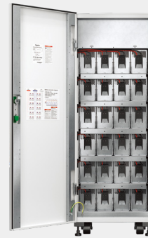
Modular battery cabinet for extended runtime requirements
