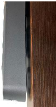
(X) A gap between the wall and the reader
