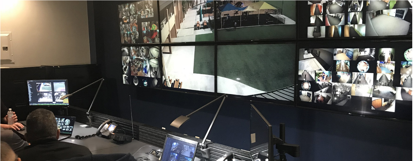
Video Wall users can create and remotely manage remote monitors with just a few clicks.
