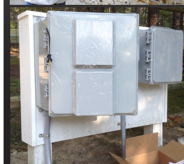
Installer made mounting surface
