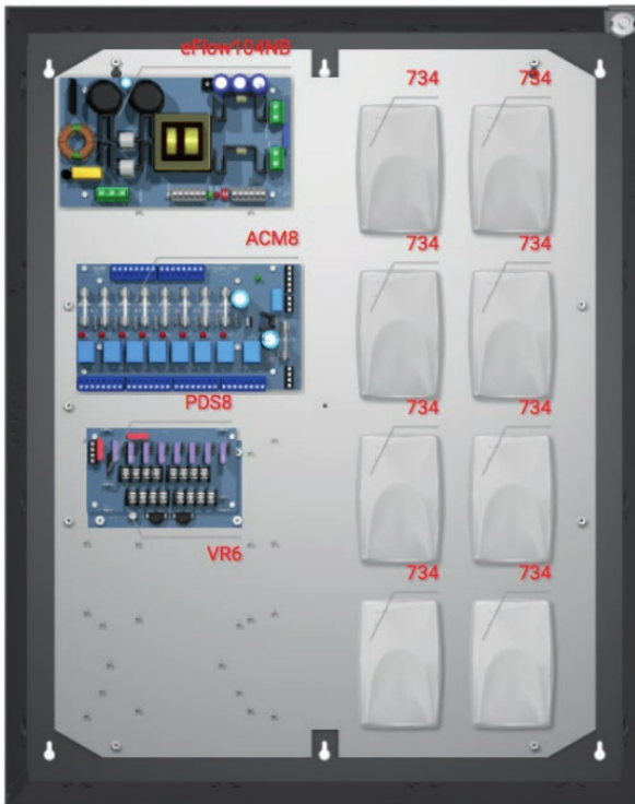
T2DMK7F8 8-Door Access System with Power
