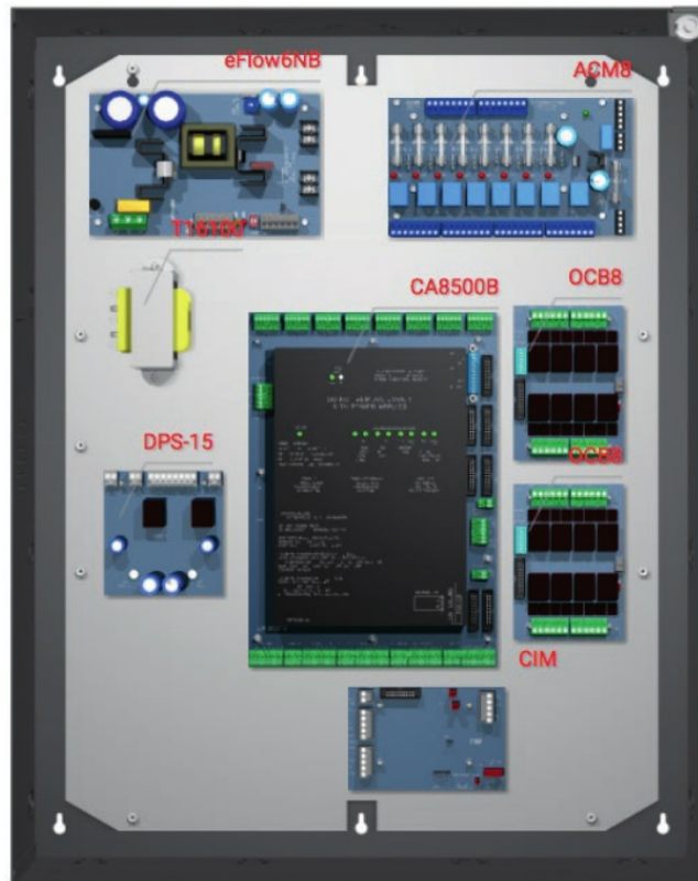
T2KK3F8 8-Door Access System with Power
