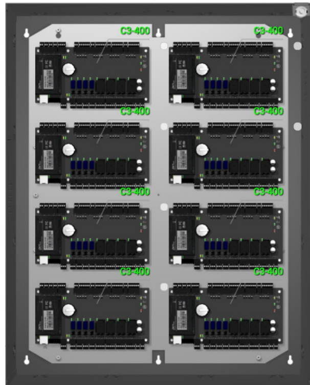
32-Door Access System
