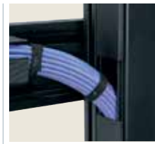
4 horizontal cable management
