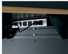
Two securely-mounted 4-outlet power strips: one mounts to the table bracket for connections close to the display and includes a cover; the other is located inside the TechPed™ for table box connections.
