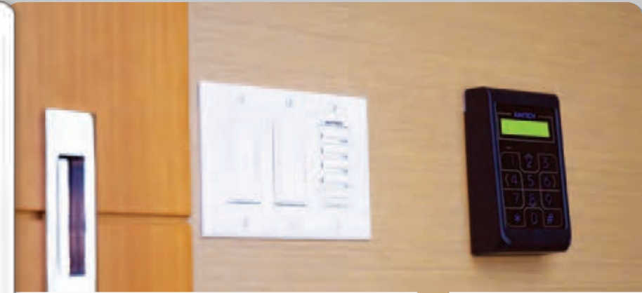
“Stand-alone proximity access control system”
